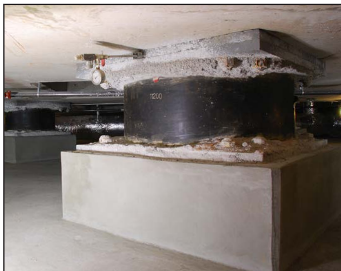
Fig. 3.5: An example of base isolation under the Utah State Capitol Building. (Source: Mike Renlund)
