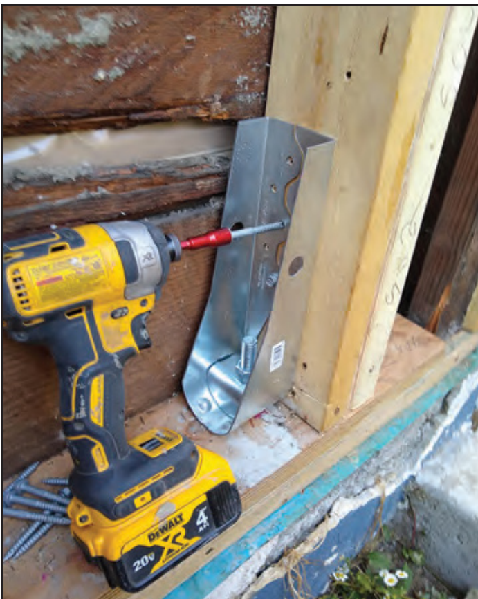
Fig. 4.4: 1270 Balmoral Rd. seismic upgrading work, partially financed by the House Grant program (Source: Victoria Heritage Foundation, 2020).
