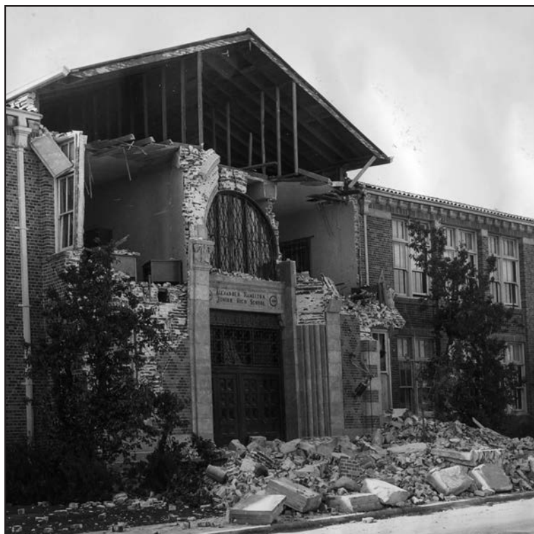
Fig. 5.5: A damaged school from the 1933 Long Beach Earthquake in California. (Source: LA Times Archive)
