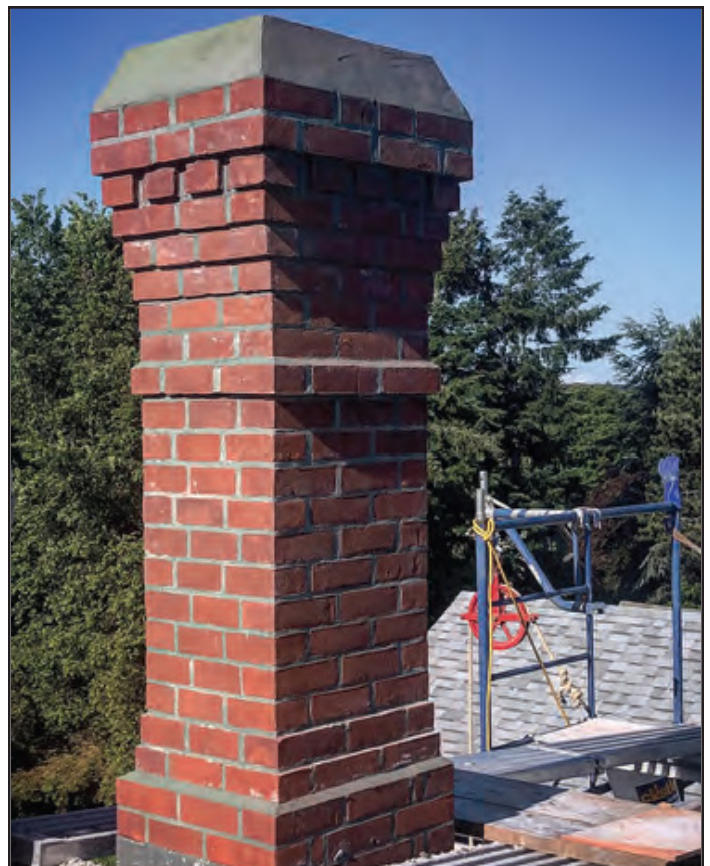
Fig. 4.5: 1260 Denman St. chimney rebuild to address its seismic vulnerability, partially financed by the House Grant program. (Source: Victoria Heritage Foundation, 2020).
