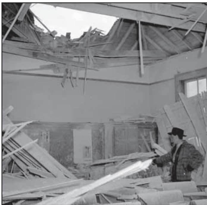
Fig. 2.6: Courtenay School earthquake damage, interior, 1946. (Source: Vancouver Public Library, 41750B)
