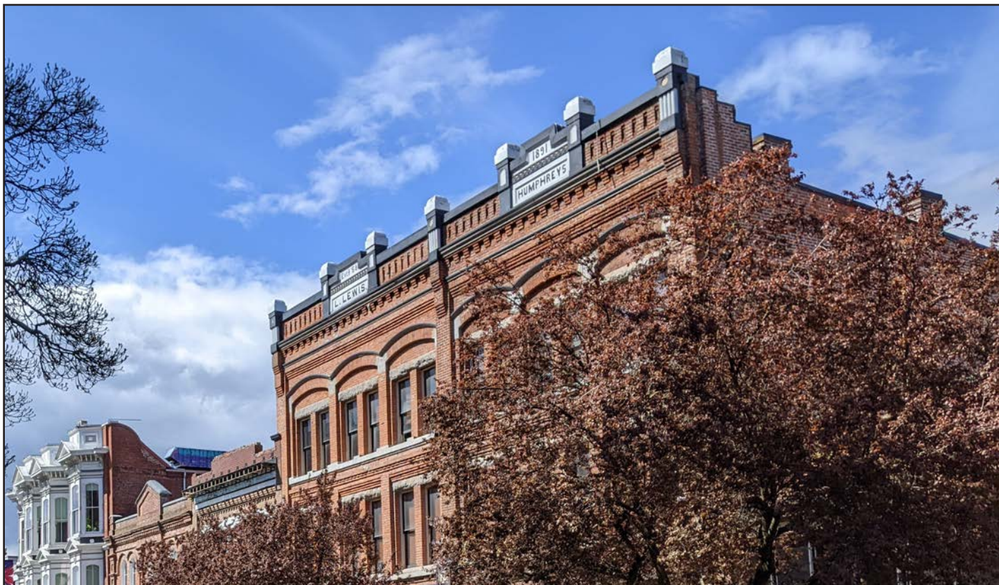
Fig. 4.7: An example parapet in downtown Victoria, BC. Such parapets, if unbraced, are at a high risk of collapse during a seismic event and would be eligible for the Seismic Parapet Incentive Program (PIP) funding. (Source: Ian Babbitt)
