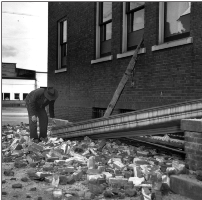
Fig. 2.4: Courtenay Post Office earthquake damage, 1946. (Source: Vancouver Public Library, 68768A)
