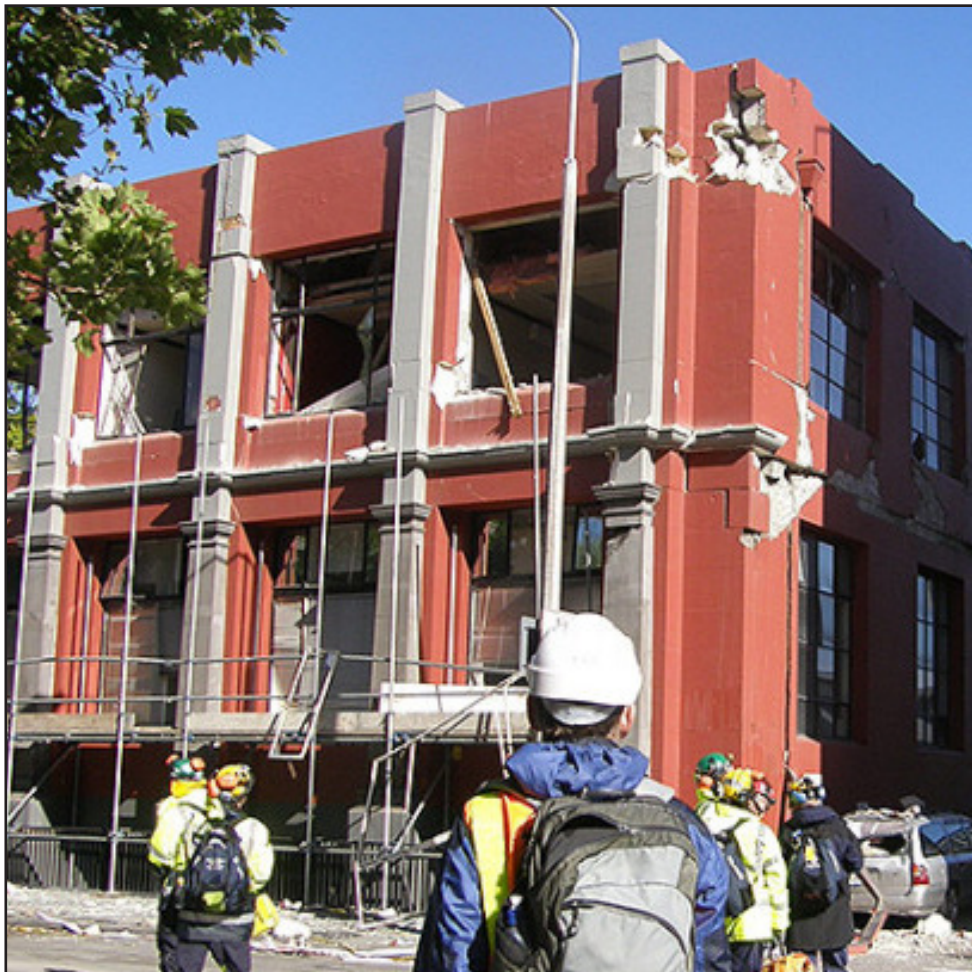
Fig. 5.24: Photograph of earthquake damage used to advertise the REPB Financial Assistance Scheme. (Source: Building Performance, Government of New Zealand)
