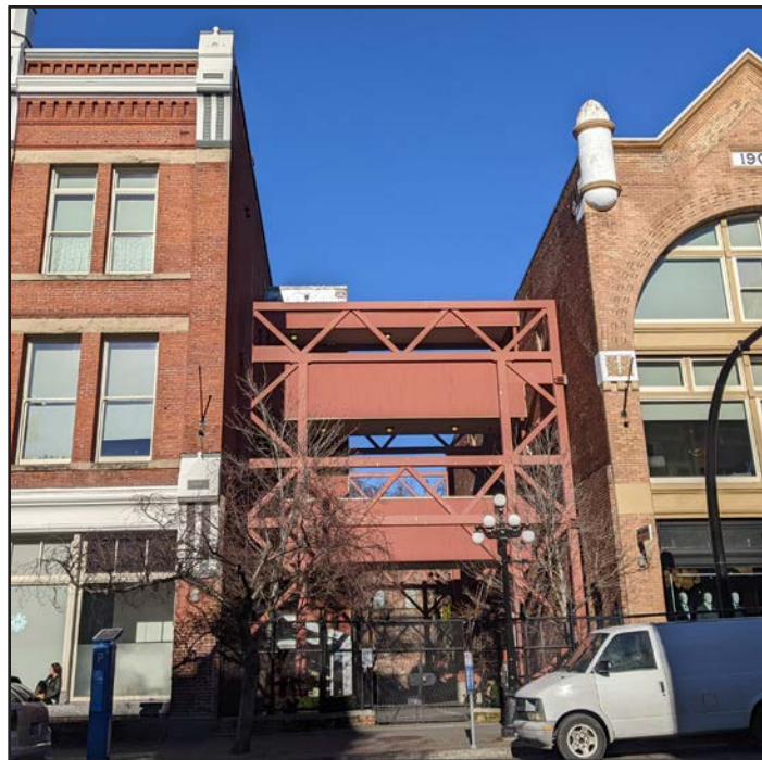
Fig. 4.6: Illustration of the bracing installed between the Leiser Building and the Earle Warehouse as part of its seismic rehabilitation work on Yates Street in Victoria, BC. (Source: Katie Cummer)
