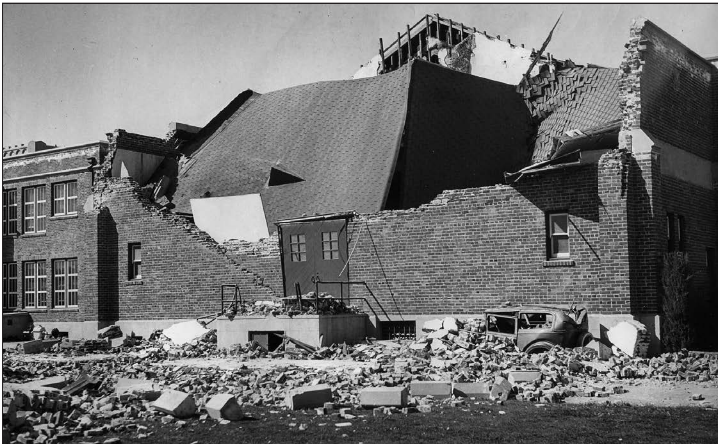
Fig. 5.6: A partially collapsed school from the 1933 Long Beach Earthquake in California. (Source: LA Times Archive)
